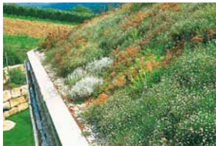
Even after only one vegetation period the plant coverage is largely complete. The roof area in this example is drained by means of an outer-lying gutter into which the three water spouts carry any excess water.
