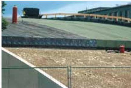
The transition area was covered with gravel and topsoil, in order to connect the roof with the natural ground underneath.
