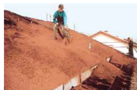
The system substrate “Heather with Lavender-light” is, e.g. delivered in a silo tanker. It is then blown onto the roof until the Georaster® elements are filled and covered up to about 10 mm over their upper edge.
