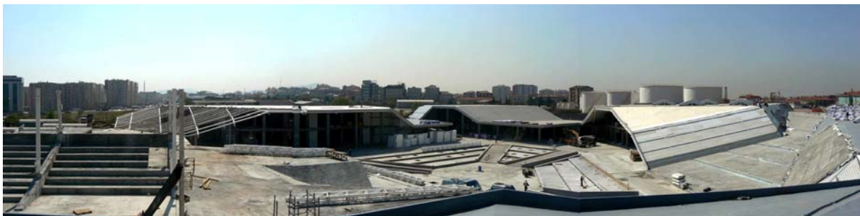
Image 2: An overview of the construction site before the green roof installation starts
