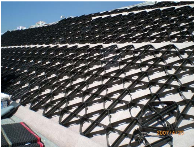
Image 5: The ZinCo-Georaster®-elements applied over the full surface provides reinforcement for the subsequently applied substrate layer
